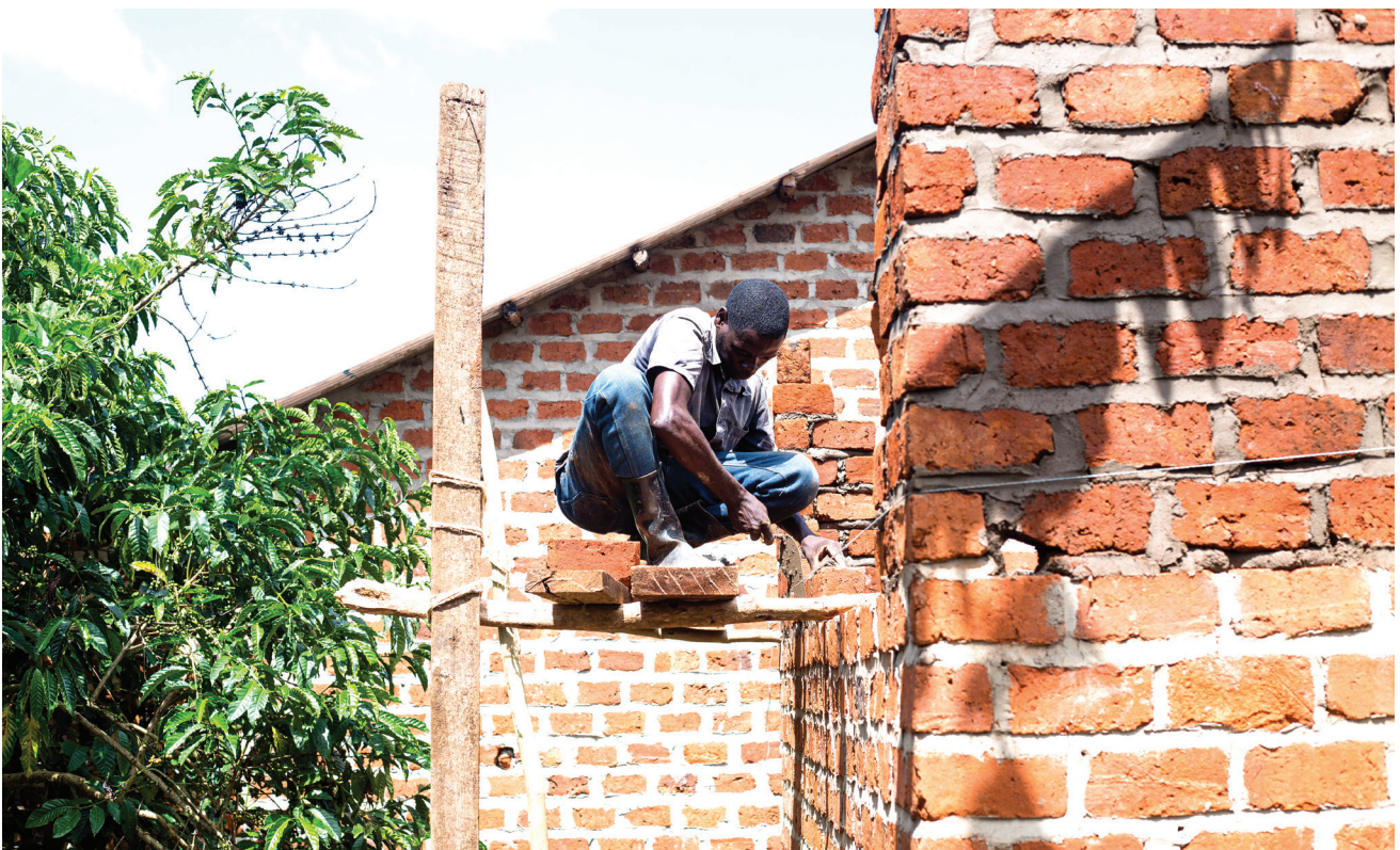
Eddy Semakula bricklaying on one of the houses built by Sapphire Africa Foundation for Nighthrose: A woman under the Sapphire Africa Foundation program for the disabled.
